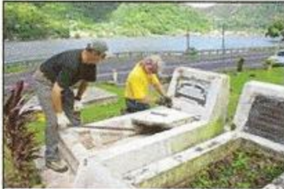
Martin Johnson (left) and Karl Munsum (right) of Monument Conservation Collaborative, a restoration company from Connecticut, seen here working to restore one of 60 grave monuments damaged by the September 29, 2009 tsunami. (Courtesy Photo)
