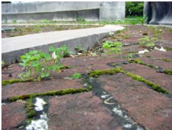
Frost heaving on brick pavers
