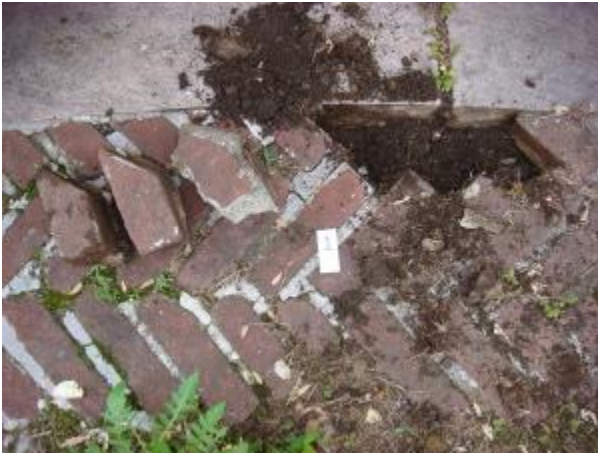
Loose paver bricks
