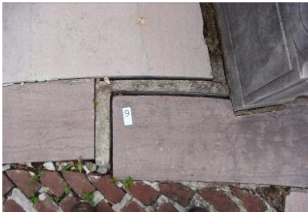
Stone movement and replacement mortar
