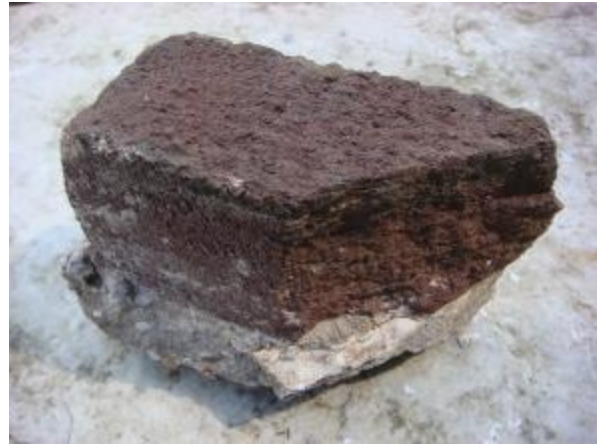
Detail of loose brick. Note setting mortar
