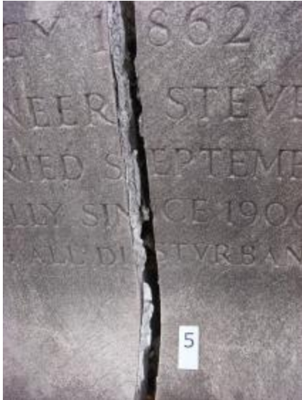
Open joints in exedra with lettering
