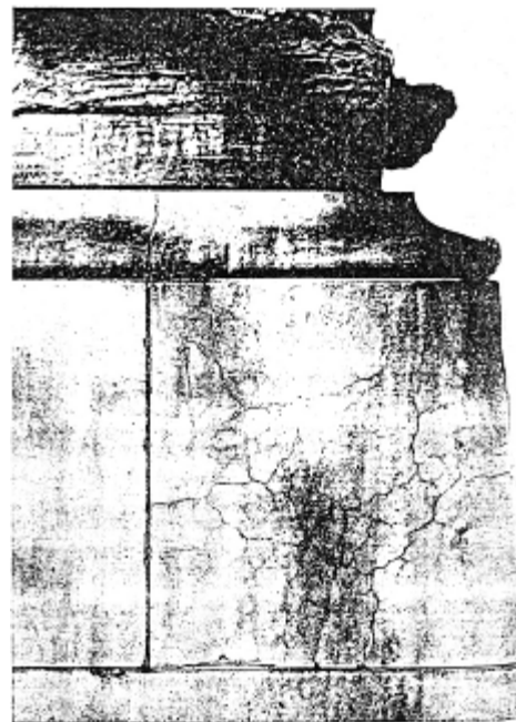
FIGURE 3. Block of badly cracked marble under the north statuary group of the Grant Monument showing the worst condition in this structure.
